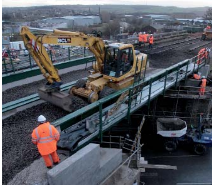
Increased work on the railways is the only positive news to come from the Workload Trends survey
