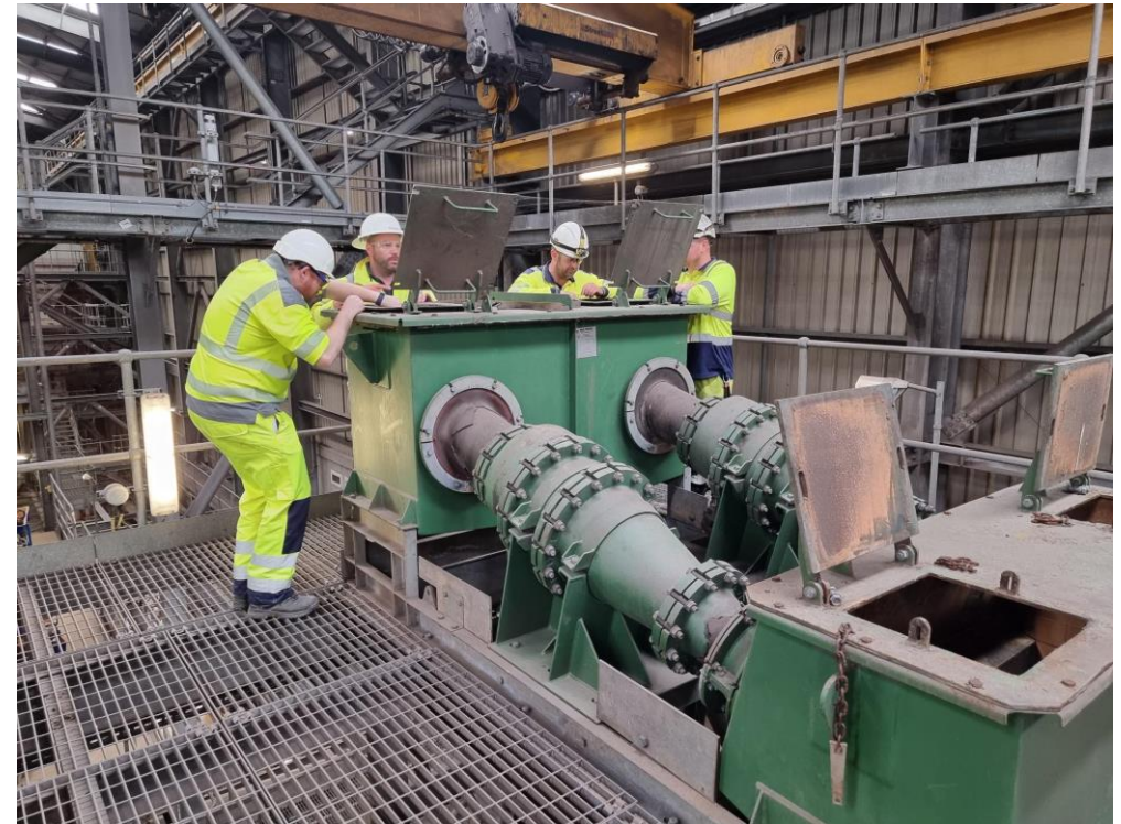
Secondary DMS to be upgraded
