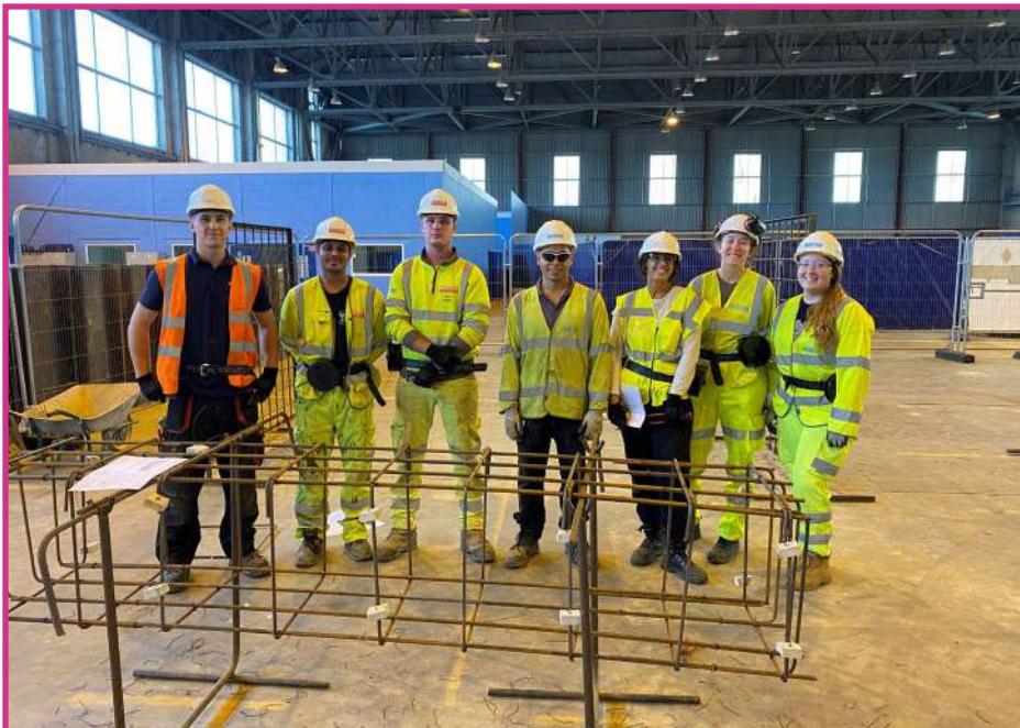
Practical Skills Week: some of our new entrants at Bircham Newton trying out their steelfixing skills
