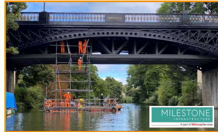
Left: Cleveland Bridge refurbishment over the River Avon in Bath by Milestone
