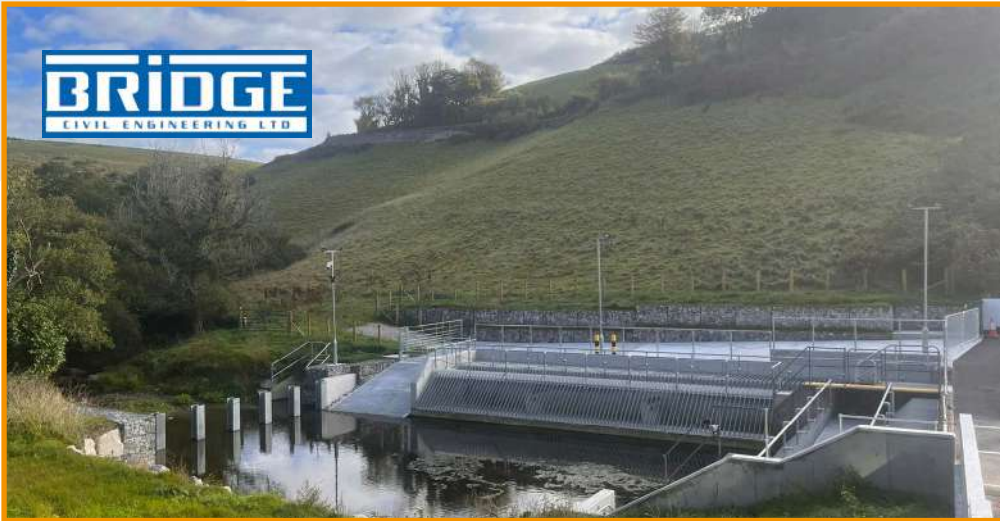
A new screen was built by Bridge Civil Engineering for the Environment Agency in Polperro in 2022
